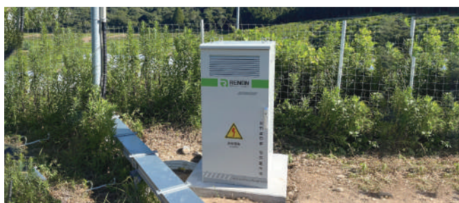
Renon DC ECube 38kWh
