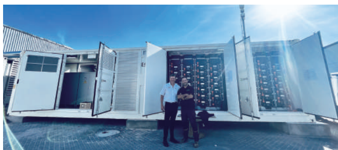
Renon Estation 744kWh
