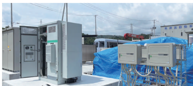
Renon DC ECube 157kWh
